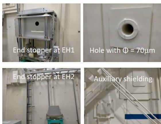
Fig. 3. End stoppers at EH1 and EH2, the hole, and the auxiliary shielding.
