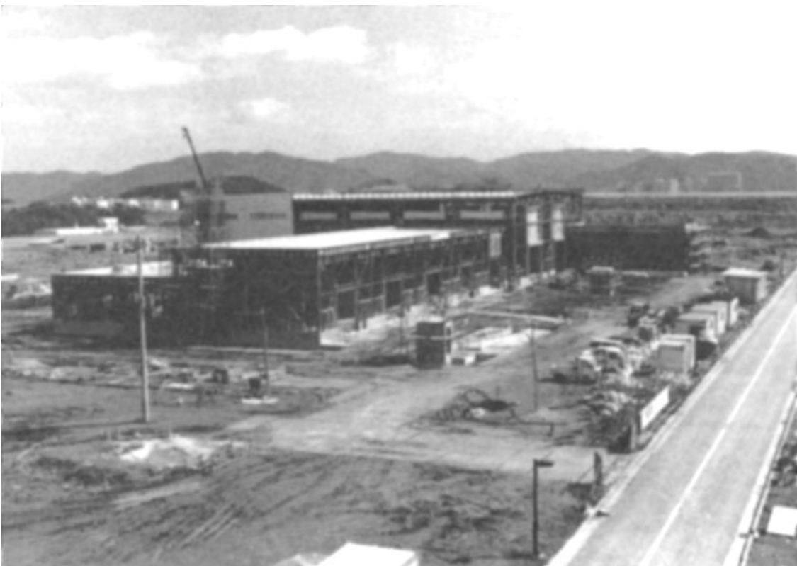
Accelerator and Beamline R&D Facility (view from the Machine Laboratory)
