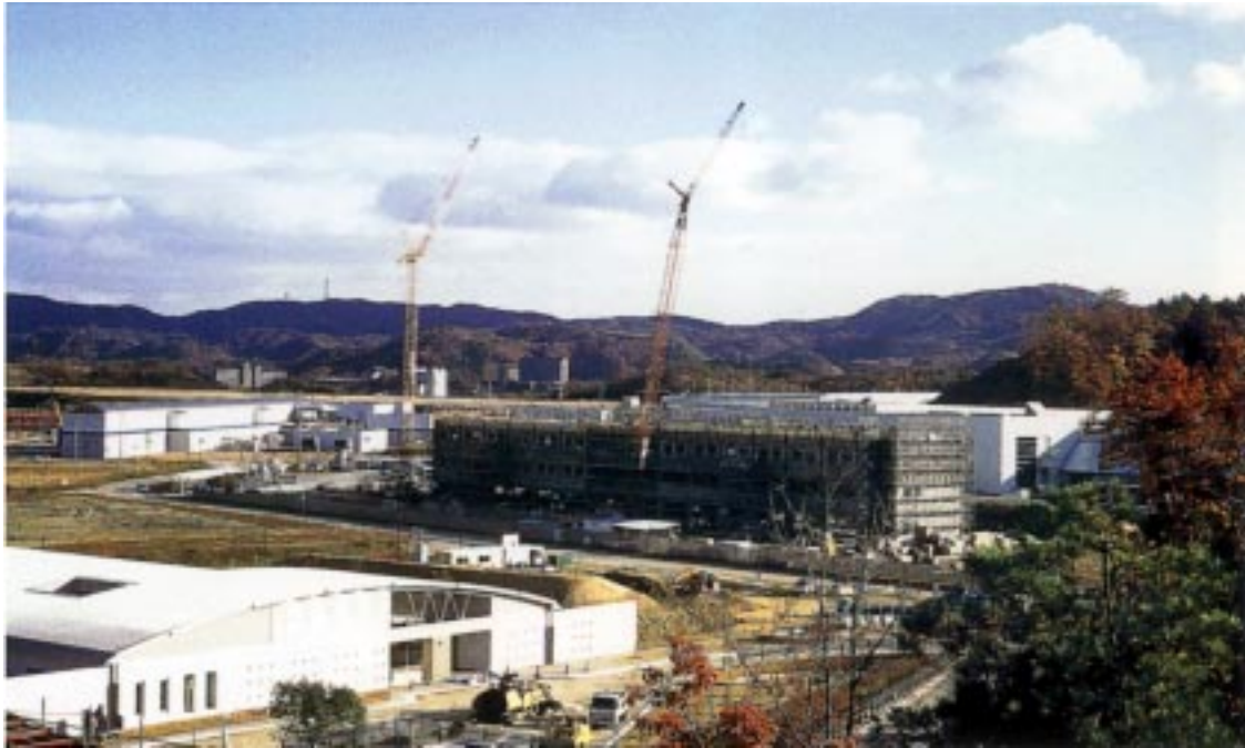
The main building (center) and cafeteria (lower) of the SPring-8 facility both under construction at the time when this report has been prepared.
