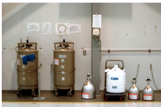
Fig. 6. Liquid Nitrogen Corner
