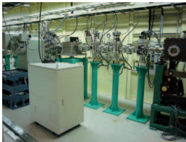
Fig. 2. Components of optics hutch. The SR beam comes from the left. The double-crystal monochromator (left), first mirror (right), and other beamline components (e.g. shutter and slit) between them can be seen.
