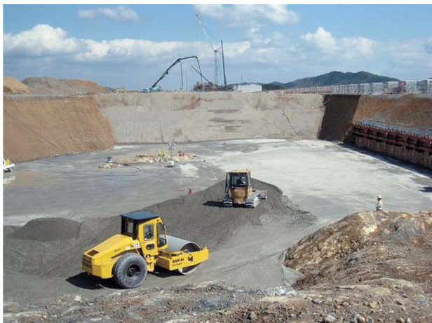
Fig. 11. Rolling procedure for forming stable and high-density artificial rock bed.
