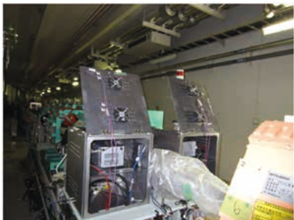
Fig. 9. Setup of power supply system in the accelerator tunnel. The power supply system is placed in the radiation and noise shield box.
