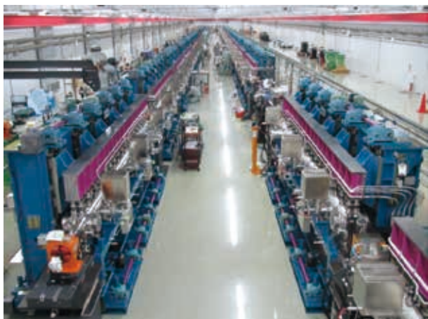
Fig. 1. New BL2 undulator line (left) installed in the SACLA undulator hall together with the existing BL3 (right).
