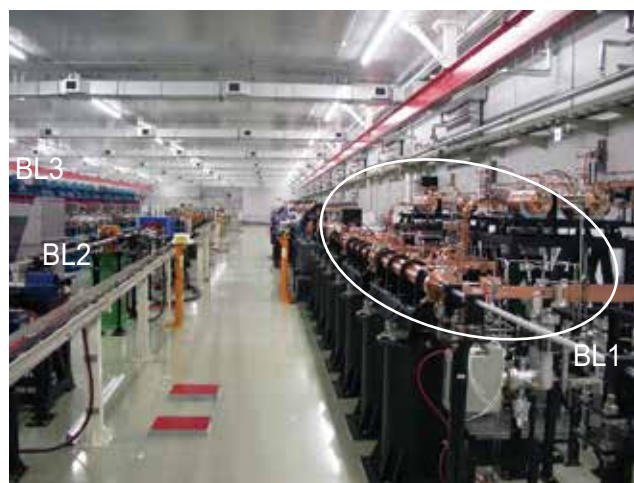
Fig. 3. BL1 to BL3 beamlines in the undulator hall taken from the experimental hall side (i.e., the downstream side) of BL1. The white circle indicates the newly installed C-band accelerator units in the BL1 accelerator.
