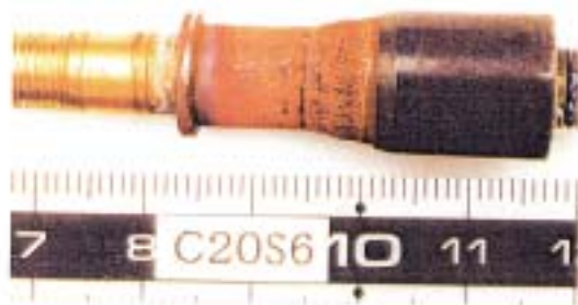
The rod of the water-flow switch in use, which made on-appropriate alarm.
